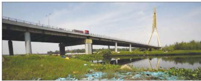
the floodplains, some of which has topped into the river bed underneath the Sarai Kale Khan flyover. There is so much debris that an active river channel is now disconnected from the main river. The debris was dumped recently
